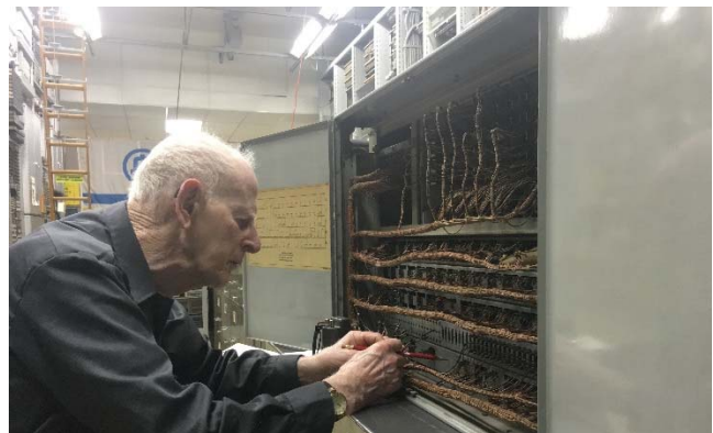
Volunteer Les Anderson works on the rear side of a terminating sender.
